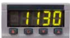
Over-temperature limit controller
