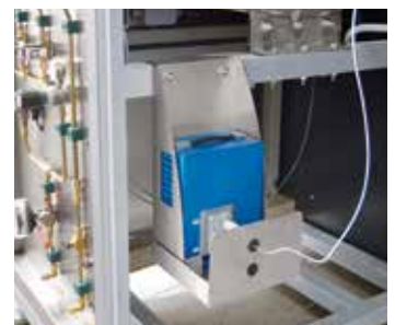
Acid pump for nitric acid
