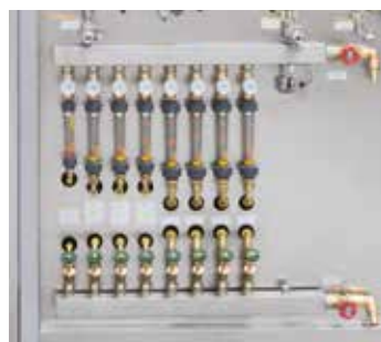
Cooling water distribution
